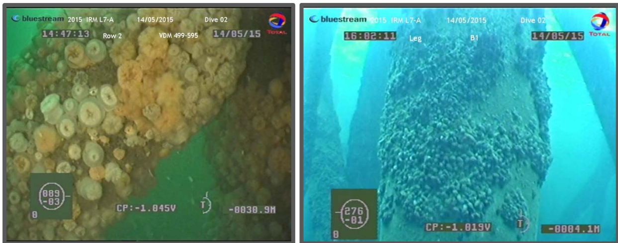
Figure 6. Fouling community on the piles of platform L7A. Left photo Metridium Senile and right photo, Mytilus edilus .
